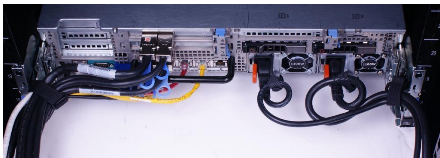
Figure 9. Cable routing without a CMA
