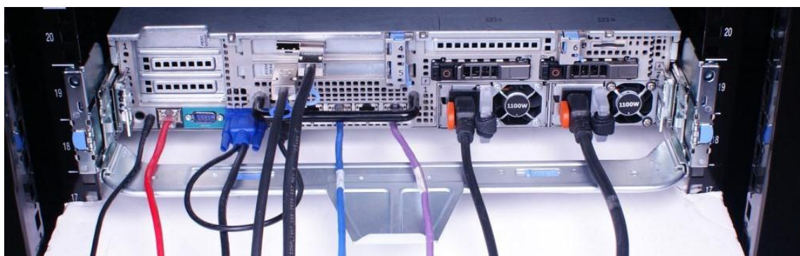
Figure 1. System with cables installed
